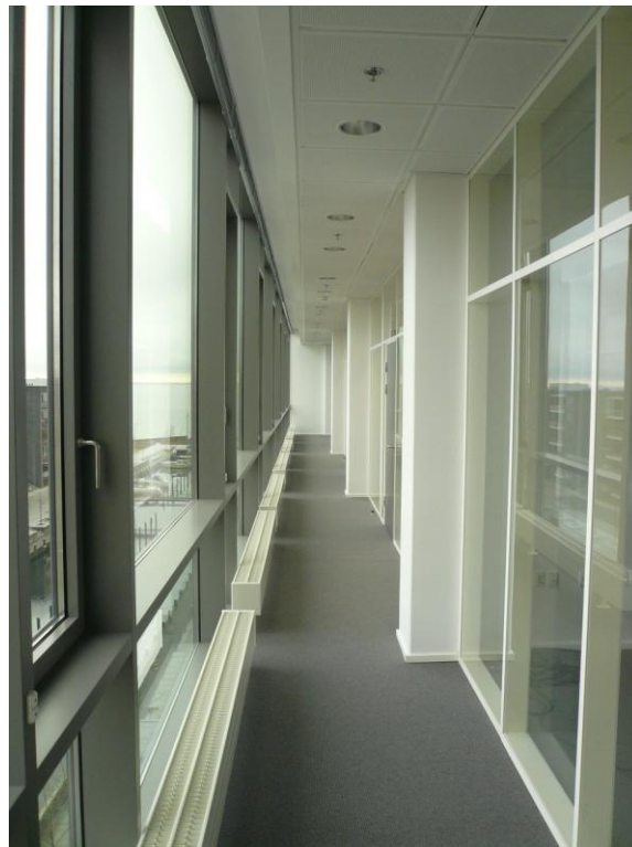
Figure 2.11. Example of a radiator along the façade.
