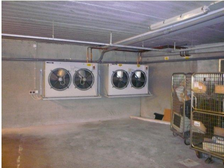
Figure 2.16. User installation in the basement for cooling server rooms.
