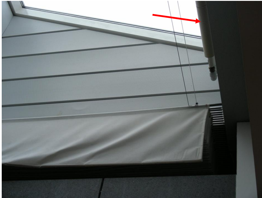
Figure 2.12. Convectors at the skylight in the atrium.
