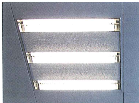
Figure 5. Built-in luminaries in the offices.
