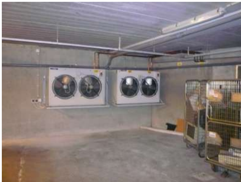
Figure 2.16. User installation in the basement for cooling of server rooms.
