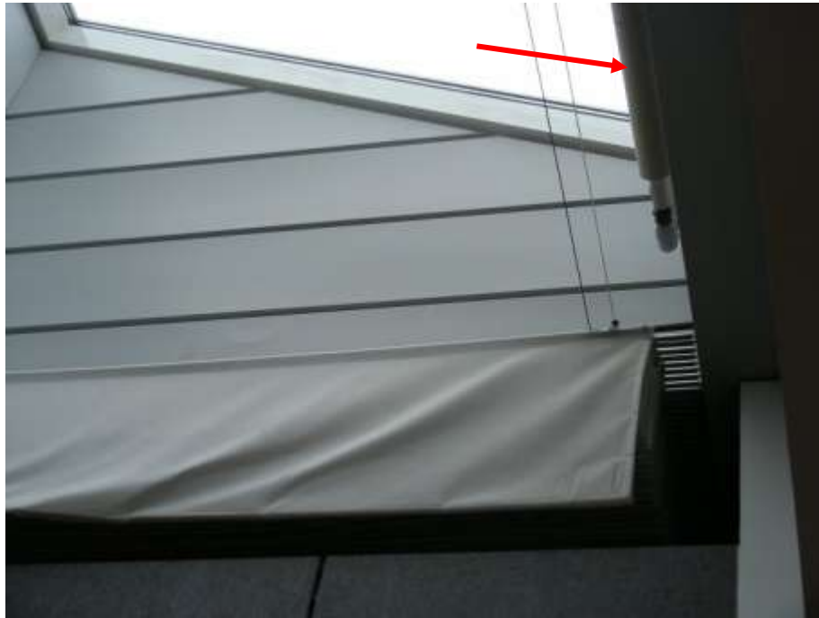
Figure 2.12. Convectors and curtains under the skylight in the atrium.
