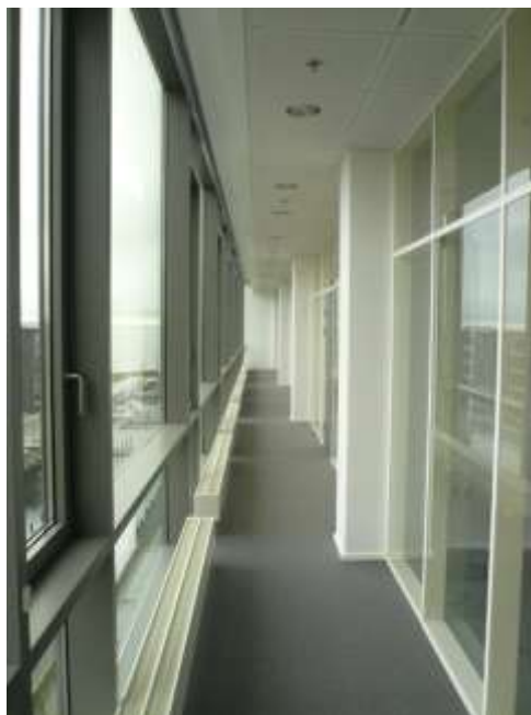
Figure 2.11. Example of a radiator along the façade.
