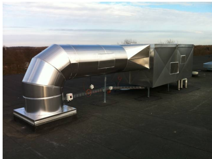
(b) Exchanger coil on the roof
