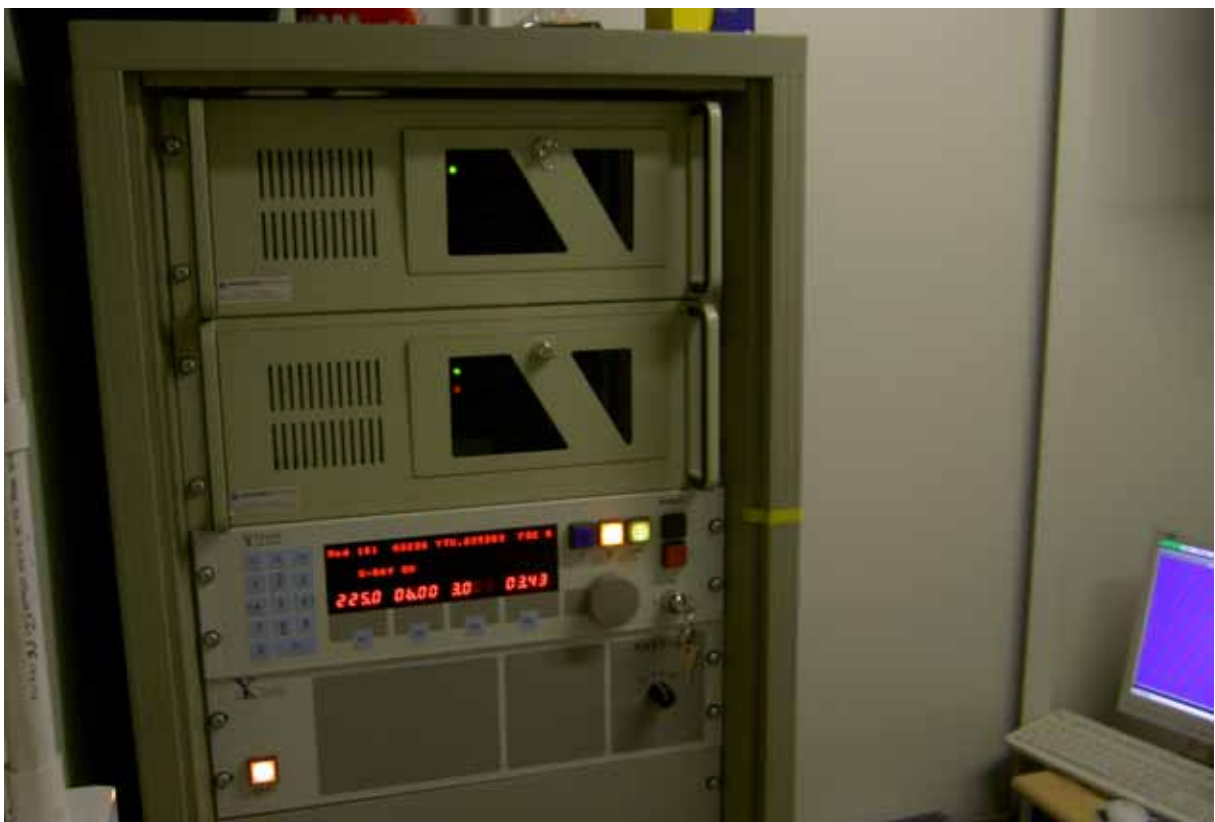
Figure 5-9 Cabinet from which the x-ray is controlled. This is where the kV and the mA for the x-ray is set. These parameters need to be adjusted considering the geometry and the alloy being cast.
