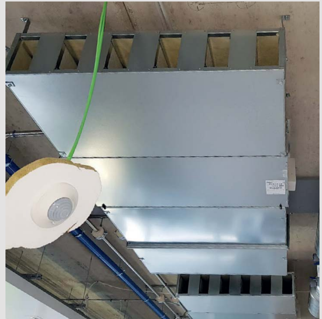
Fan Coils mounted over the ceiling
